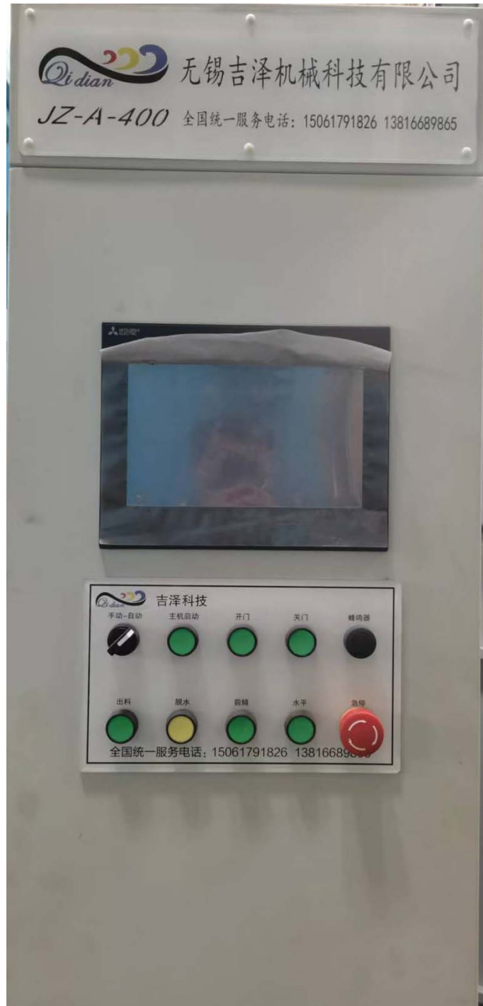
P4 Electrical Cabinet
