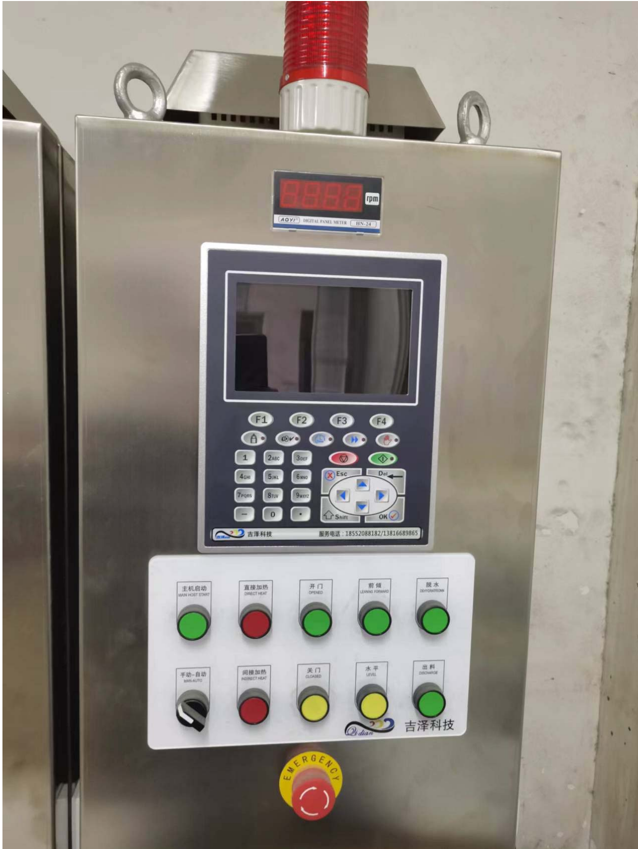
P4 Electrical Cabinet
